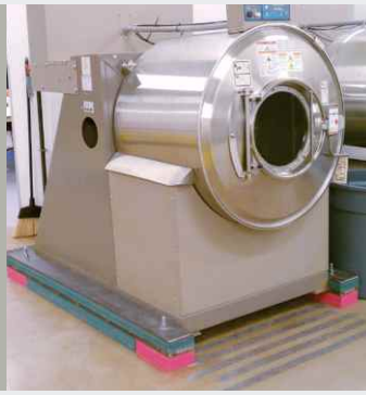
Elastic decoupling of an industrial washing machine
