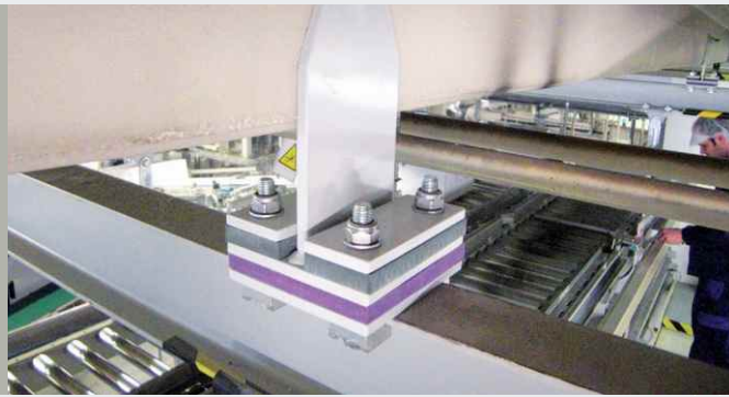
Elastic decoupling of a production plant for food
