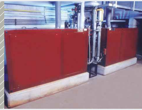
Elastically mounted combined heat and power plant
