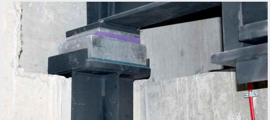
Double elastic bearing using Isotop® SE-DE, overhead cable guide
