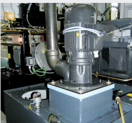
Decoupling of a pump with Sylomer® and Sylyodyn®
