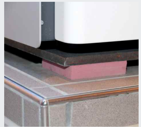
Elastic decoupling of an indoor unit with Sylomer® discrete bearing
