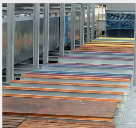
Bearing of an air-handling unit on Sylomer® strips
