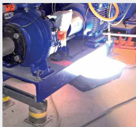
Pump bearings without additional mass (foundation) with Isotop® DZE
